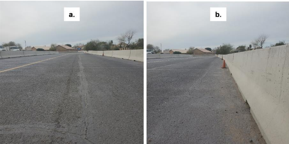
Figure 23. CP-B Section – March 2023; a. Wheel path; b. Shoulder.
