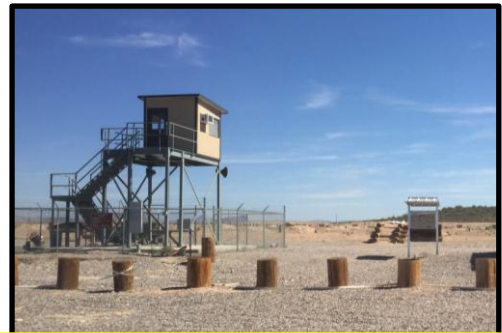
Existing structures will need to be analyzed and strengthened accordingly to increase the probability of surviving a large storm. Photo taken by researchers.
