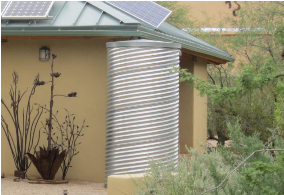
Figure 35 Residential rainwater harvesting system installed at a home in Tucson, by City of Tucson
