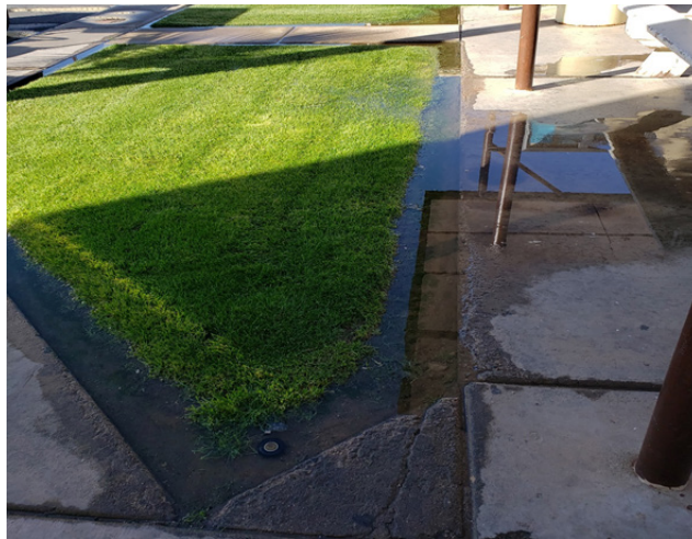
Figure 38 Water pooling and leaching, which is not approved for greywater use
