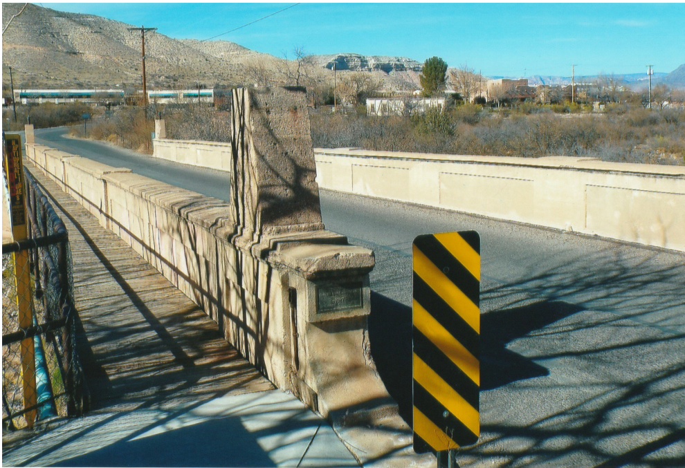
Figure 2 Current state of Bitter Creek Bridge, via Wikimedia Commons at https://commons.wikimedia.org/wiki/File:Clarkdale-Broadway_Bridge-1917-2.jpg
