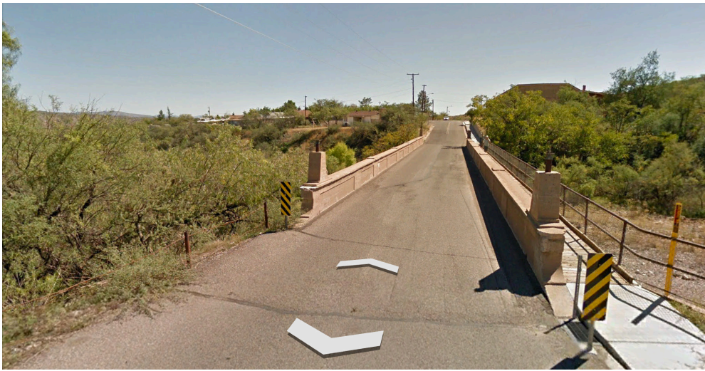
Figure 7 Bitter Creek Bridge south-facing view, showing concrete details and added pedestrian access, from Google Earth
