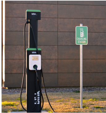
Figure 9 Blink IQ200 Level-2 chargers
