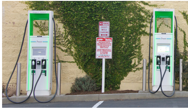
Figure 10 DC Fast Charging Stations
