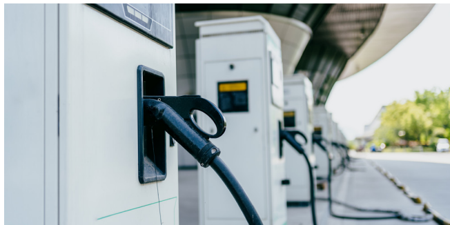
Figure 6 DC Fast Charging Stations
