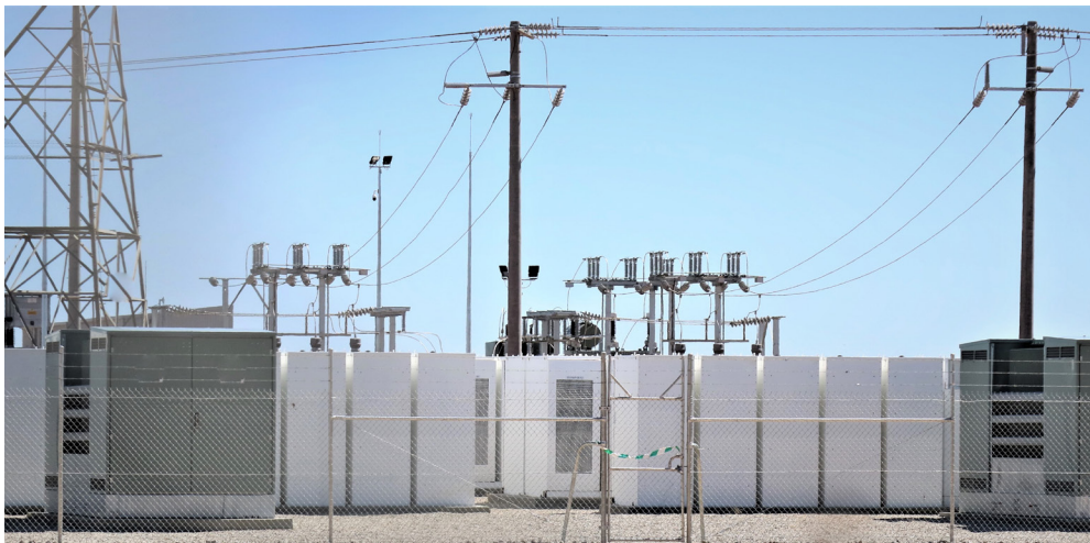
Figure 1 Battery energy storage at a solar farm
