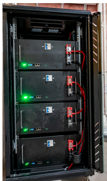
Figure 2 Bank of electric batteries in a residential home used in conjunction with a solar energy system or for backup power
