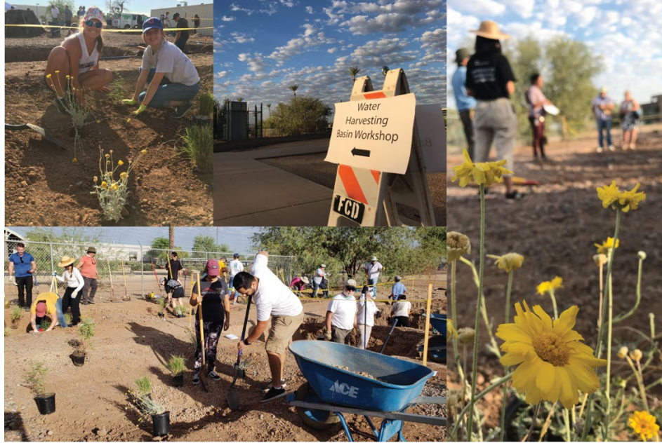
Figure 2.32: Water harvesting UEI designed experiment basins were installed with the help of over 30 volunteers made up of CAP researchers, students, Watershed Management Group members, and other helpers at FCDMC (September 15, 2018).
