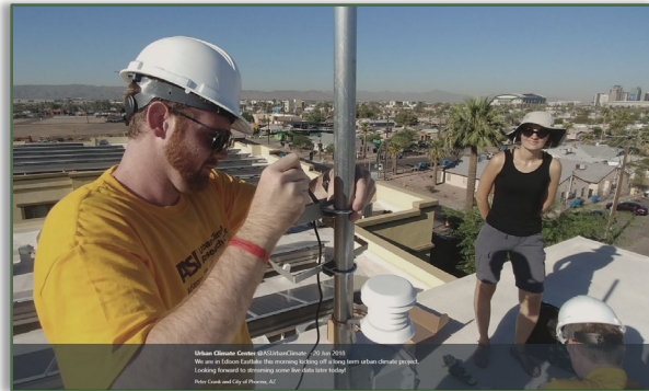
Figure 2.16. Peter Crank and Yuliya Dzyuban installing a rooftop weather station in Edison-Eastlake
