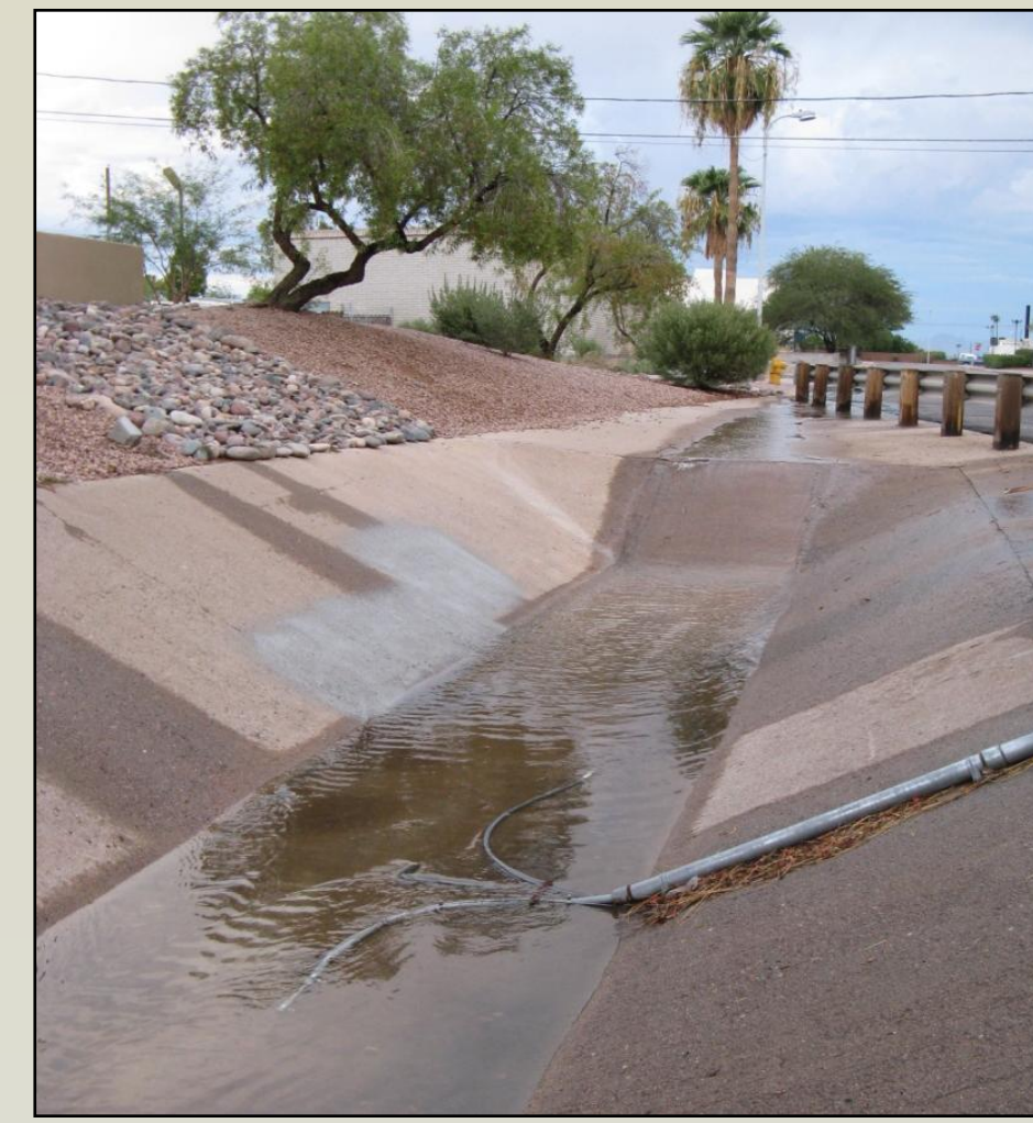
Figure 1. Street stormwater infrastructure
