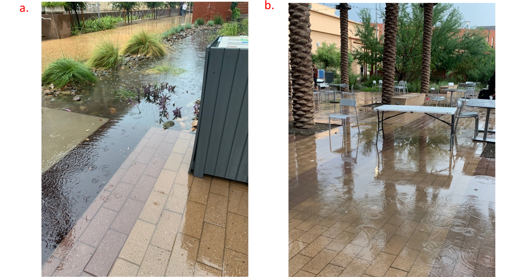
Fig. 3. a) Overflowing basin after heavy precipitation events from July 24-26, 2021. b) Example of water accumulating on impervious surfaces in Orange Mall.
